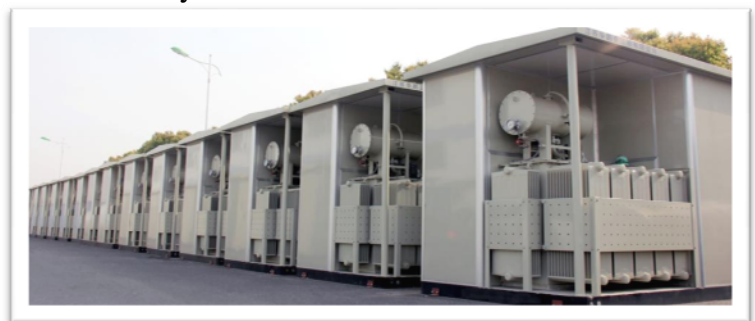
Compact Substation Design
